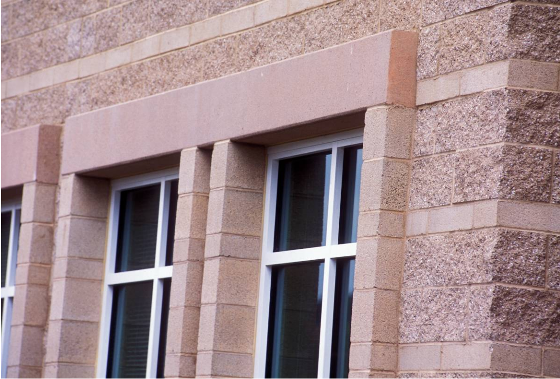
The Sun MicroSystems building is an example of how single-wythe concrete masonry construction can be aesthetically pleasing. Photographer: Jackie Schumacker, 2002.
